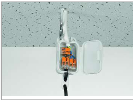
Pendant light connection in suspended ceilings
