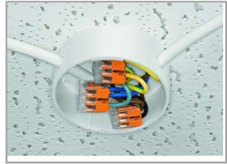
Lighting distribution in ceiling canopy
