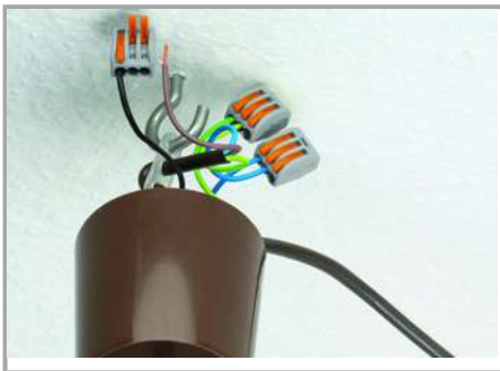
Lighting fixture connection with fine-stranded wires and power feed
