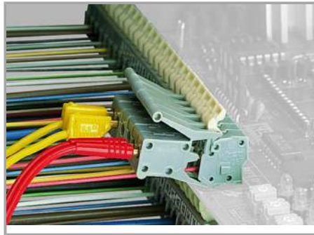
Testing with test plug modules.
