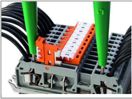
Testing with voltage tester.
